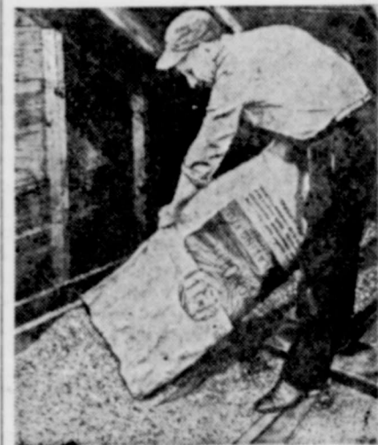
Zonolite vermiculite insulation being installed over ceiling of dairy barn at Sinissippi Farms, Oregon, Ill.
