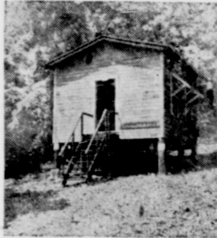
Panama test house. This photo shows that treated wood had not been attacked by termites.
