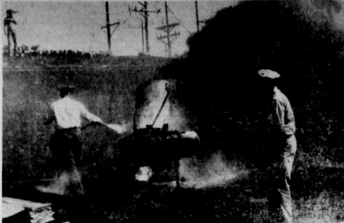
OVER-HEATED tar pot bursts into flames today and damages structure of new home being built by Clyde Dungan at 606 S. Thirteenth St. (Advocate Photo)
