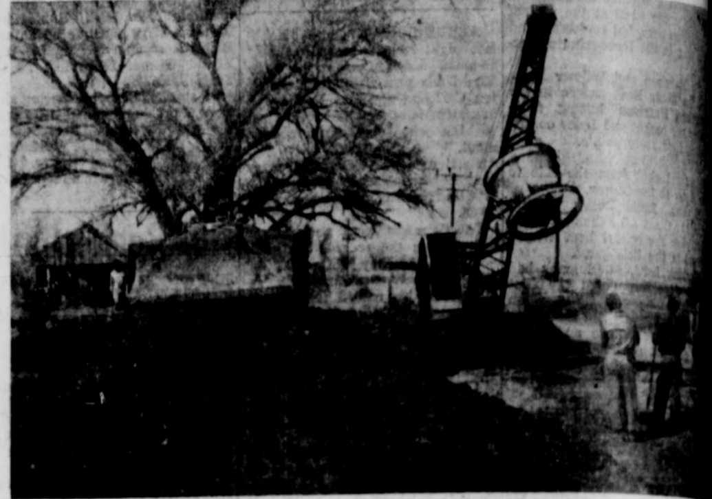
A DITCH LINING MACHINE straddles a ditch on a raised fill while a bucket crane prepares to lift mixed concrete up to the ditch liner which is too high for a mixer truck to pour into. (Advocate Photo)
