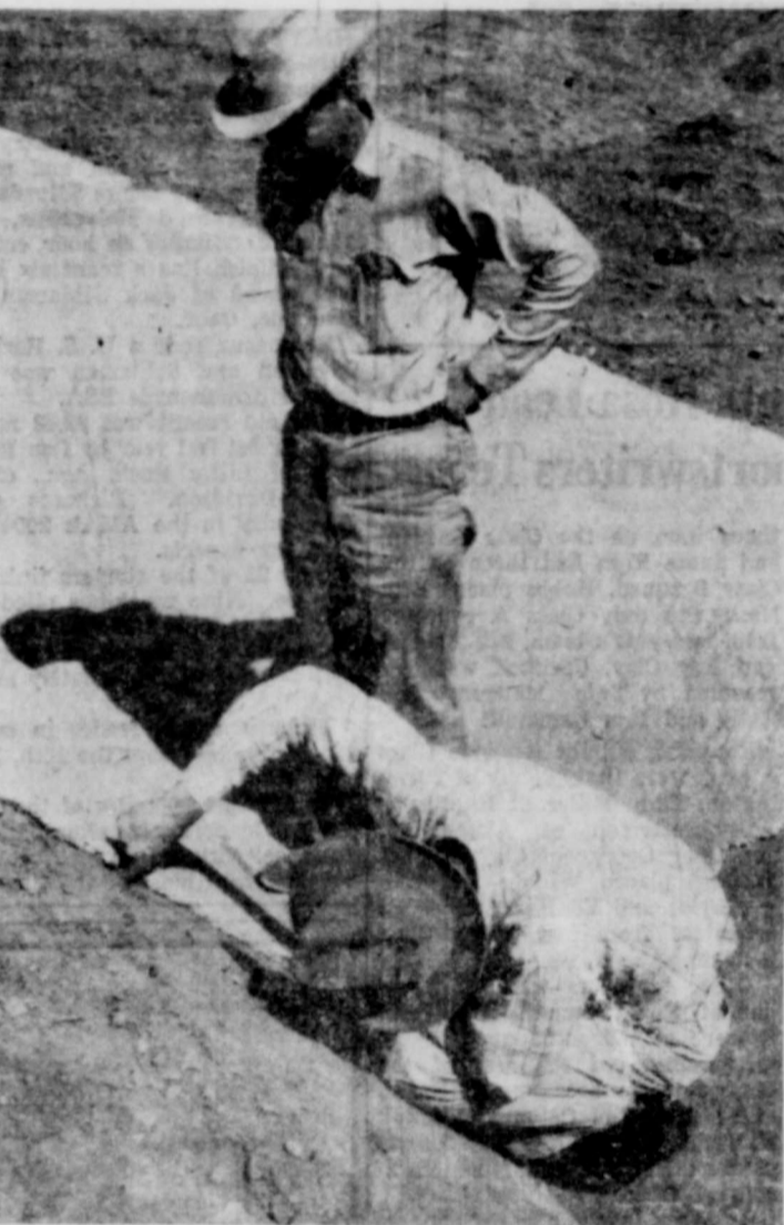
SCS ENGINEERS Bill Fox, standing, and Doug Henson, examine the concrete lining job on one of the irrigation ditches at the Bill Langenegger farm. (Advocate Photo)
