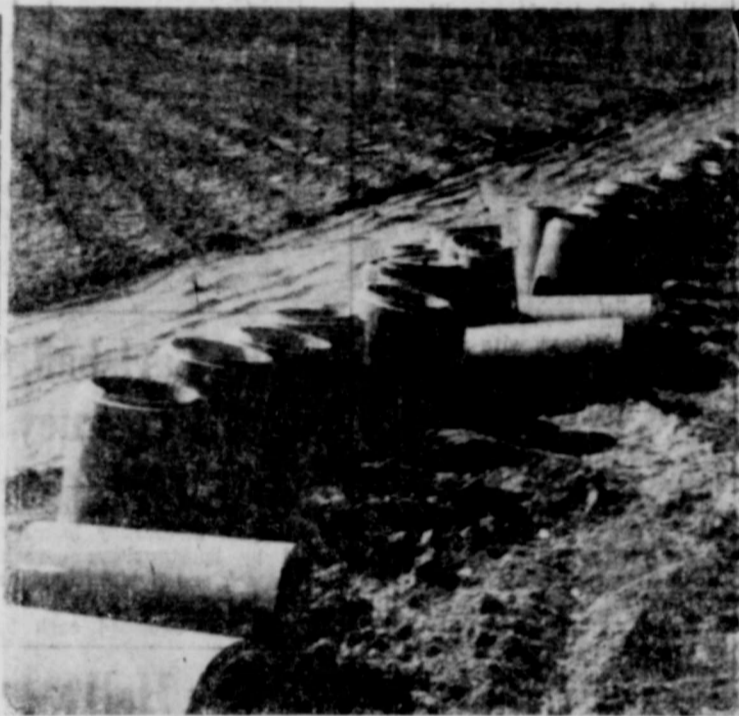
UNDERGROUND CONCRETE pipe will siphon water under pressure from pumps at the wells to the irrigation ditches, which are on a higher level than the well outlets. (Advocate Photo)
