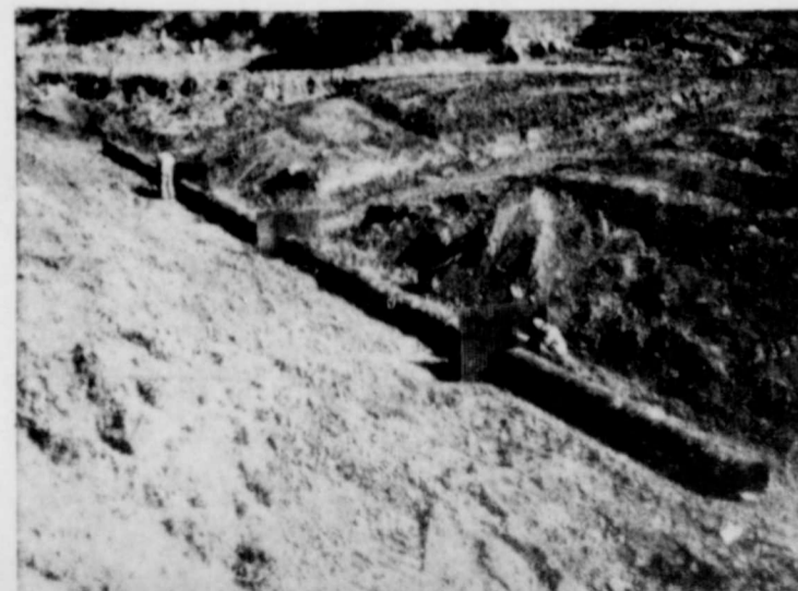
LAYING OF DRAIN PIPE during construction of No. 10 check dam on the Pearson Ranch.
