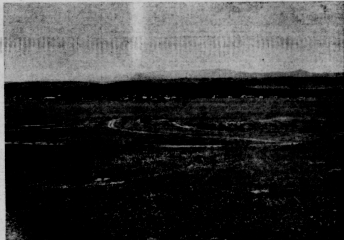
A LARGE, wet-rolled, dam at the head of a gully on the Pearson Ranch, designed to hold back runoff and prevent further cutting of the gully below.
