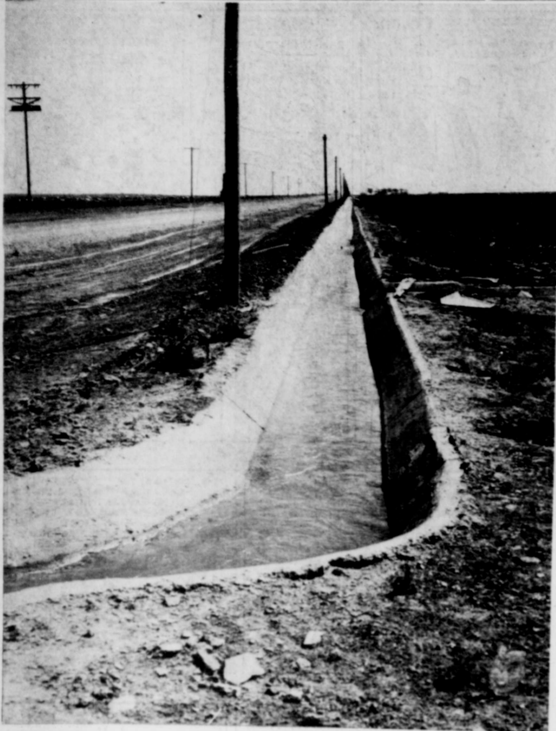
CONCRETE irrigation ditch on the Roy Ingram farm, is three-quarters of a mile long, represents continuing trend toward this type of water-saving installation in North Eddy county. Evaporation loss is very small compared to earthen ditch, and water moves fast to whatever part of field operator wishes. (Soil Conservation Service Photo)
