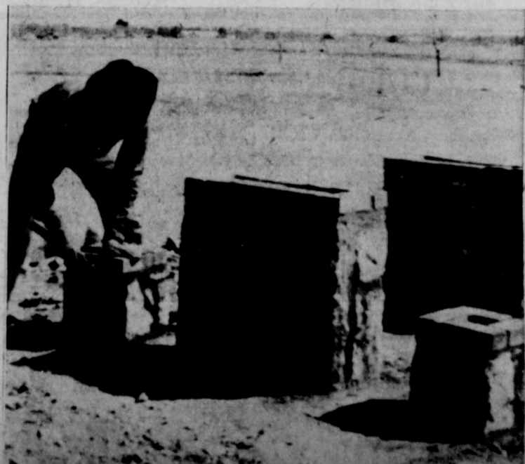
CITY PARKS offer facilities, such as stone tables and benches at Municipal Park (shown above when under construction), at all people of Artesia, includes seven parks in system.
