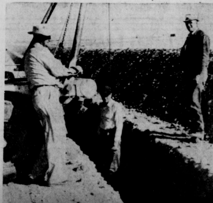
LAYING pipeline from the new reservoir west of town was supervised by water department Head L. M. "Red" Vaughn, right. Taking a break for a minute are, left to right, J. E. Chaney and Bill Fowler.
