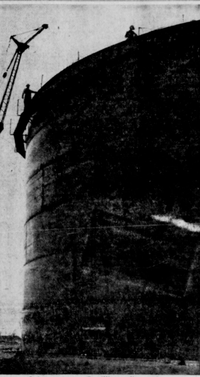
STEEL SHEETS to complete the top of Artesia's new 2-million gallon water reservoir west of town were being swung to the top of the 80 foot structure yesterday by the giant side-arm tractor, shown in picture. The reservoir tank, as far as the steel construction, should be completed by the end of this week. (Advocate Photo)
