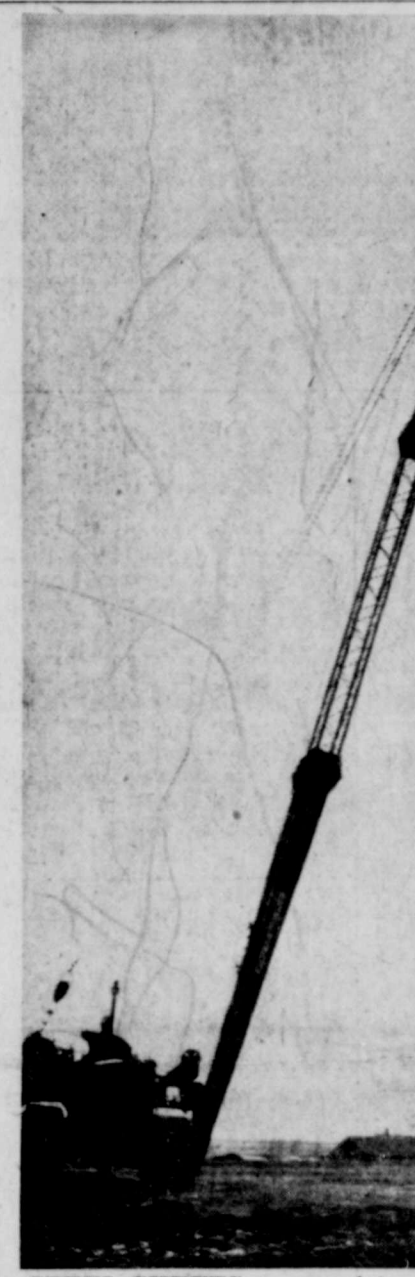
STEEL SHEETS to complete the top of Artesia's new 2-million gallon water reservoir west of town were being swung to the top of the 80 foot structure yesterday by the giant side-arm tractor, shown in picture. The reservoir tank, as far as the steel construction, should be completed by the end of this week. (Advocate Photo)
