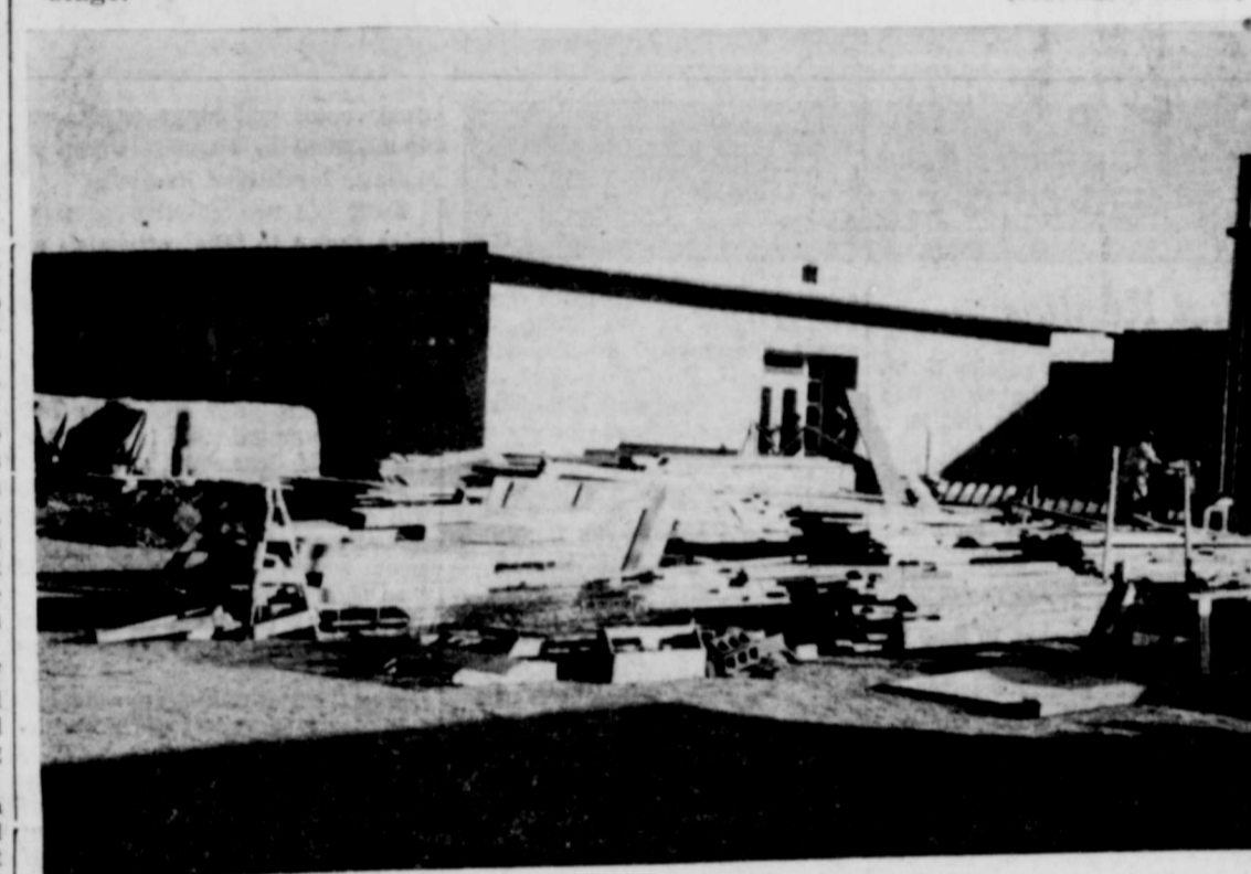
CONSTRUCTION for a 12-room addition at Junior high school has started this month, with completion date listed as Aug. 1, 1955, when 90 students will be enrolled in the school. Brickwork on the building will start Jan. 1 if weather permits. (Advocate Photo)
