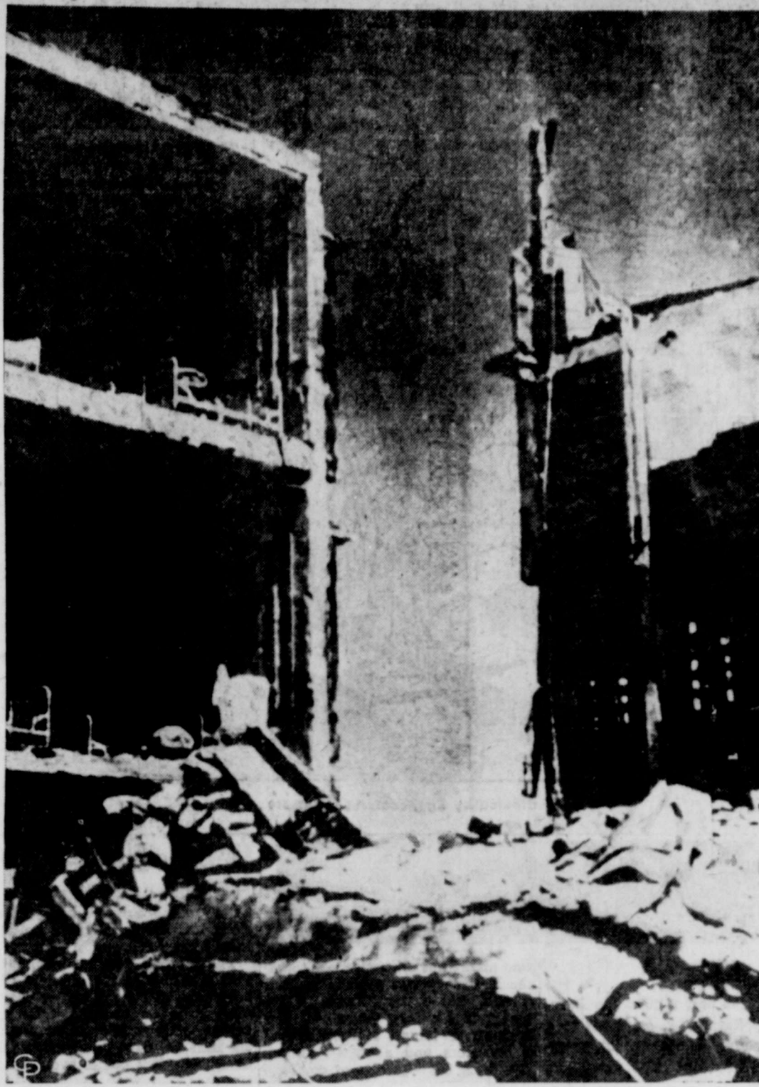
UNMUSSED BEDS make a grim silhouette in a Modern college dormitory, derailed by the North African earthquake in Orleansville, Algeria, hardest hit by the savage tremors. Official estimates place dead at 1,000, injured between 5,000 and 6,000, homeless 20,000. (International Radiophoto)
