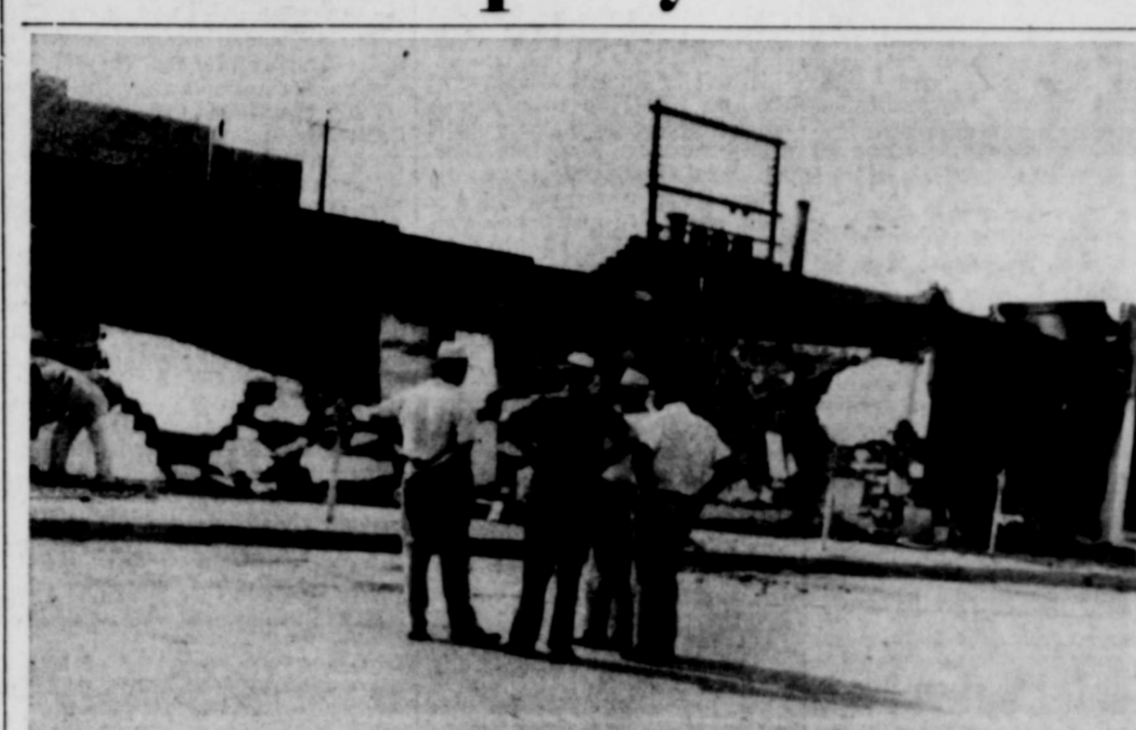
WORKMEN MONDAY demolished walls of ruined Artesia Pharmacy to prevent their collapse. Owner Ralph Petty said the property is a "complete loss." (Advocate Photo)
