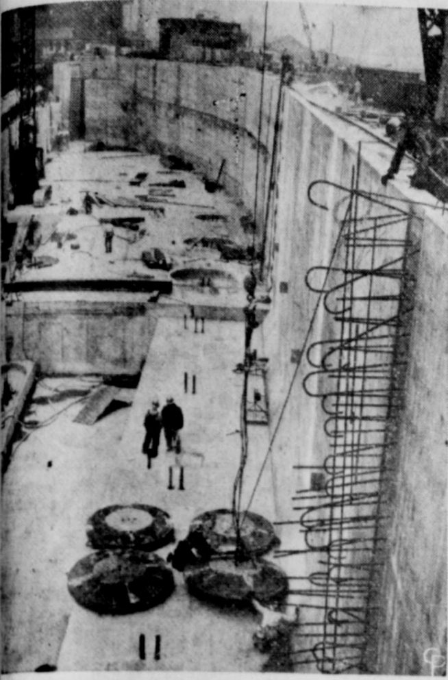
HOVE STEEL DISCS which will support steel girders of the 41-story Presidential building in Chicago are shown about to be put in place. The discs or base plates, are craned into place. About 31,000 tons of structural steel will be built into the framework by American Bridge, a United States Steel division.
