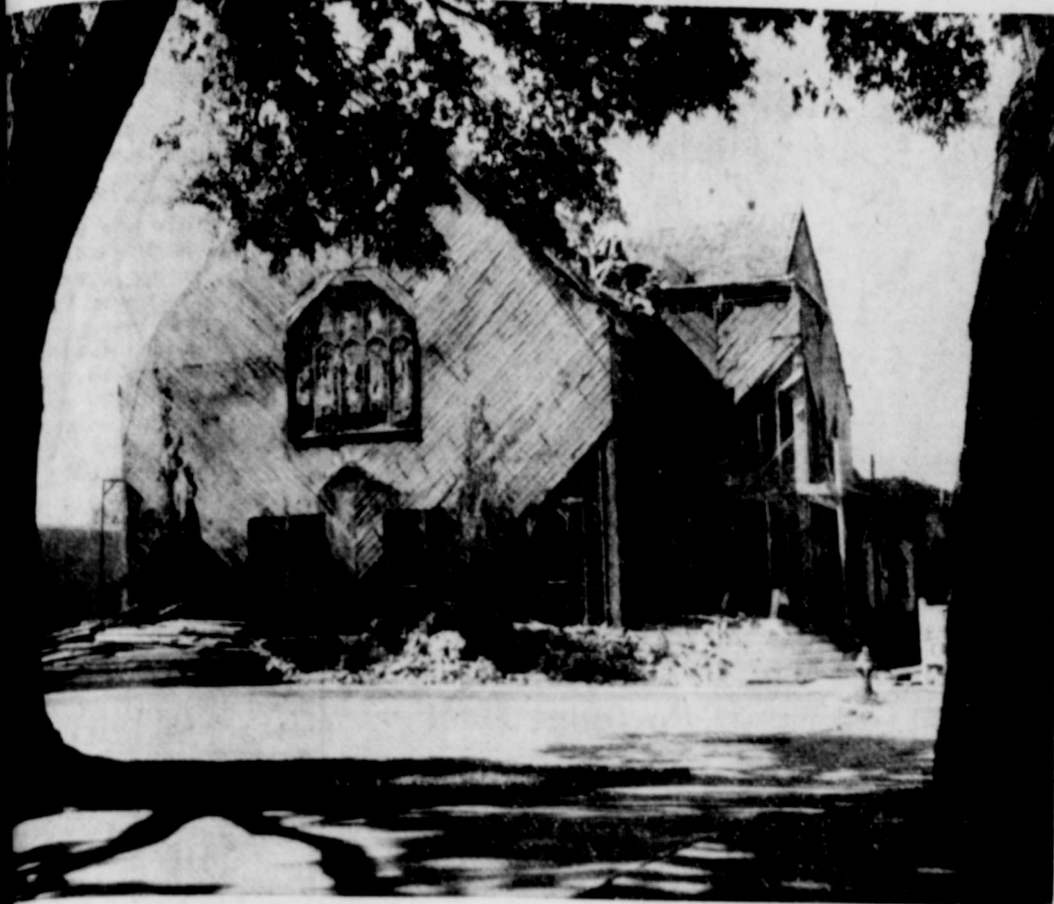
FIRST BAPTIST church is being demolished by workmen. Stripped of its exterior several weeks ago, the church is now being torn down by workmen. When razed the structure, one of Artesia's first, will be replaced by a two-story building. (Advocate Photo)
