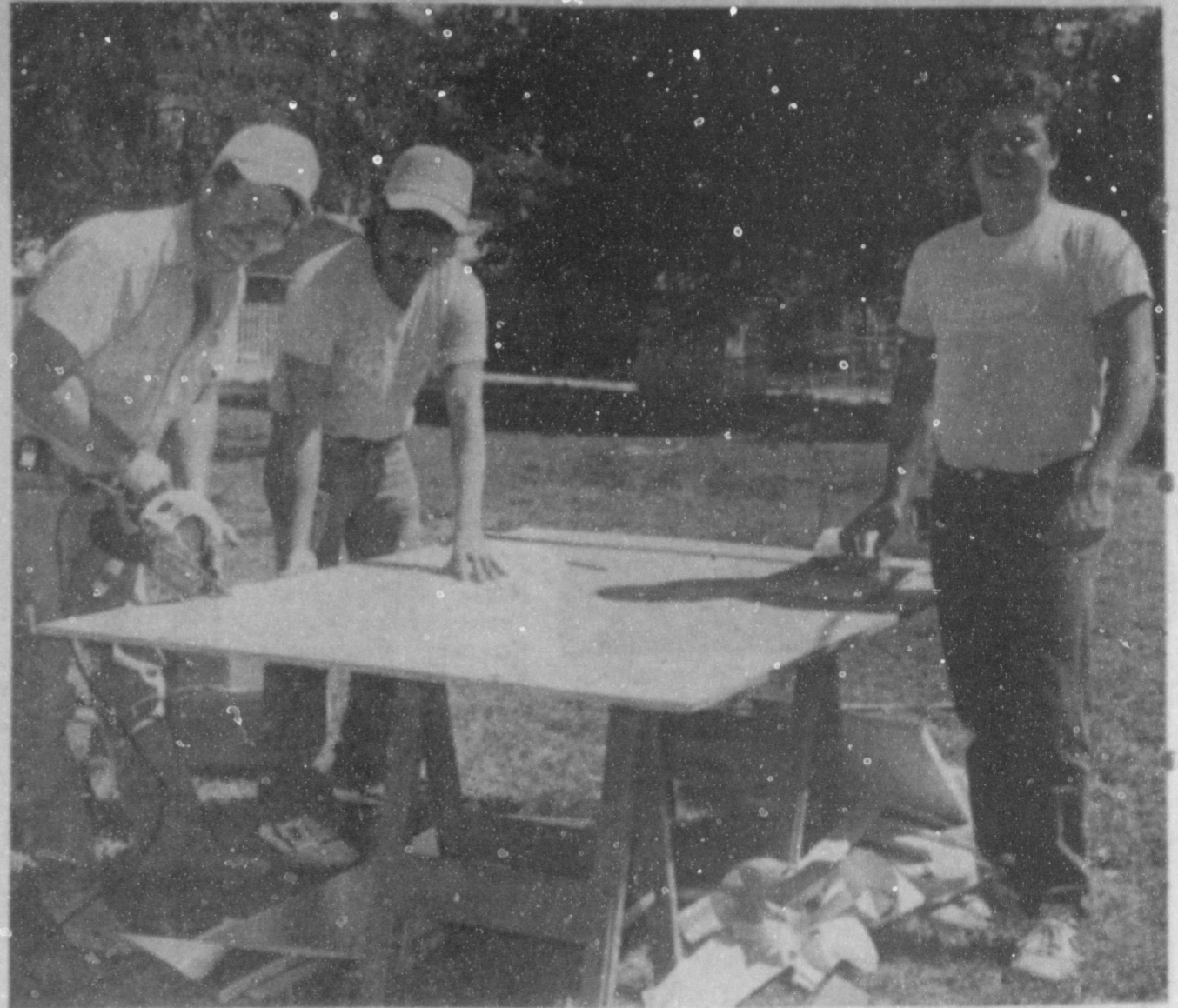
GETTING READY TO INSTALL NEW HEATING/AIR CONDITIONING UNIT AT GIRL SCOUT LITTLE HOUSE--Tuesday afternoon, employees of Plains Heating and Air Conditioning of Littlefield and Lubbock, were in Muleshoe to install a new heating/air conditioning unit at the Girl Scout Little House on West Second St. Pictured from left are Daryl Hawkins, Tony Alvarado and Pat Dillon. The new unit, and labor to install the unit was donated by Darrell Ellyson, owner of Plains Heating and Air Conditioning. He was presented a certificate of appreciation by representatives of the Muleshoe Girl Scout organization. (Journal Photo)
