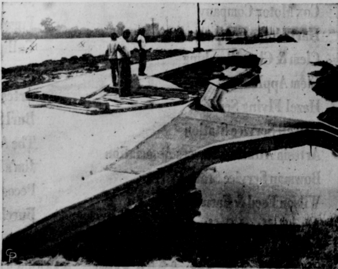
THIS IS A SAMPLE of the aftermath of havoc left in St. Charles, Mo., as Missouri river flood waters recede. Concrete north half of U. S. 40 is torn out for 300 feet, with roadfill washed away for another 500 feet. This is where power lines to St. Charles were almost washed out. (International Soundphoto)
