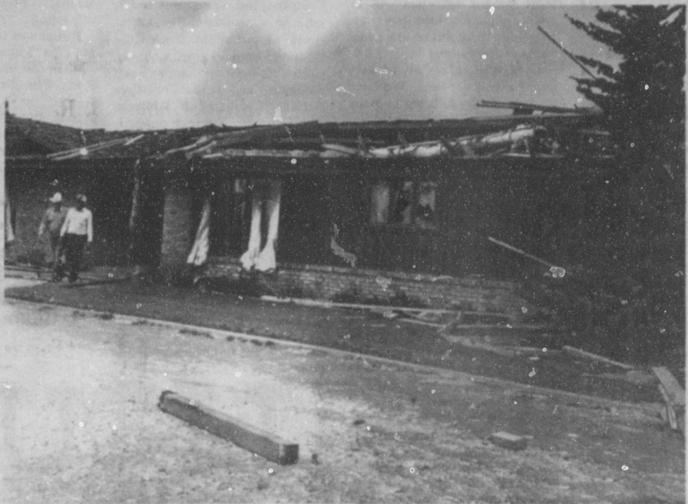
J. D. CAGE HOME FROM THE FRONT --Around 6:30 p.m. last Saturday, the J. D. Cage home just east of Muleshoe on Highway 70 literally 'exploded' on being hit head-on by a devastating tornado. This shows just a portion of the damage from the front of the home. (Journal Photo)
