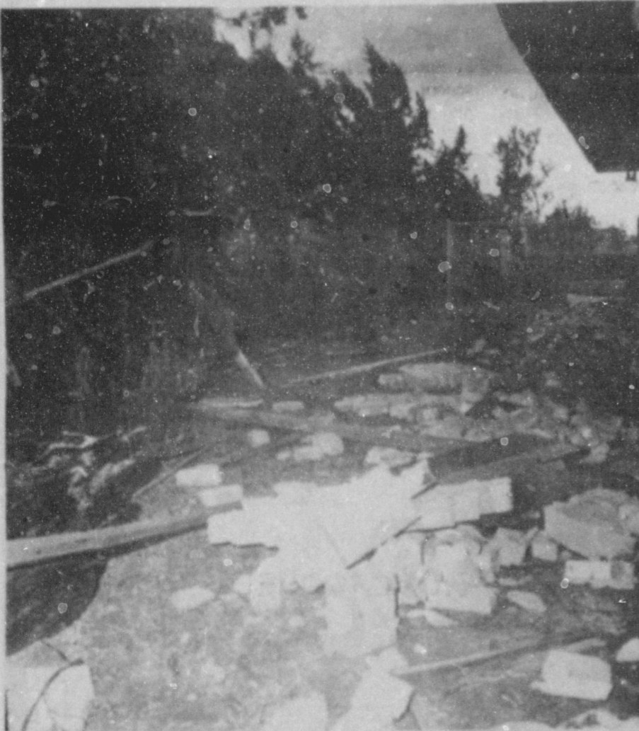
BULGING WALLS AND DEBRIS --The west side of the J. D. Cage home lost a lot of brick and lumber in Saturday's tornado. What was left of the brick wall of the house was bulging outward. (Journal Photo)
