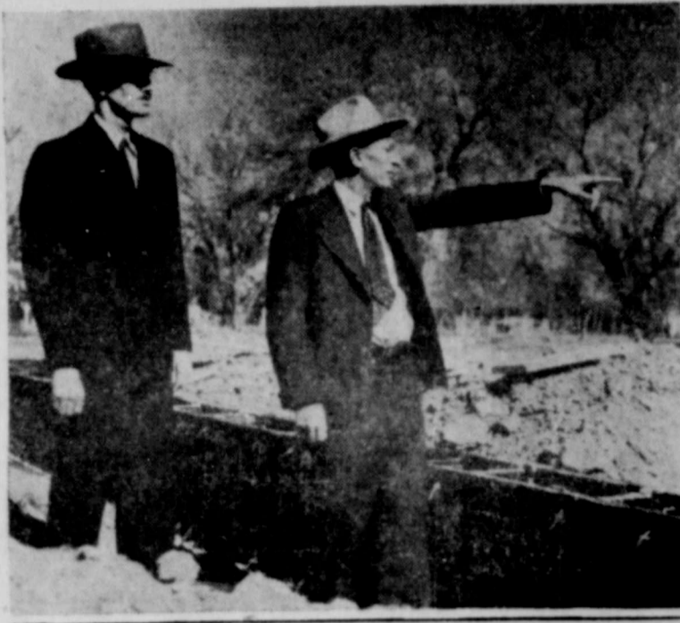
"AND THERE WILL BE THE BACK," says Albert S. Curry, associate director of the Experiment Station at New Mexico A&M College, as he points out features of the $180,710 Cotton Ginning Laboratory to Assistant Dean of Agriculture P. W. Cockerill. The laboratory, to be officially known as the Southwest Branch Cotton Ginning Laboratory, is located south of the A&M poultry farm. It will be 72' x 120' with a first floor, mezzanine, and second floor. The laboratory is being constructed by C. H. Leavell & Co. of El Paso, and will probably be completed in late summer or early fall of next year.
