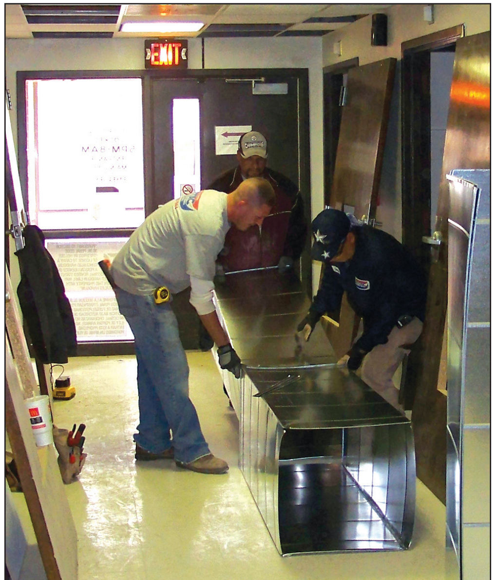
Pictured above, the construction crew works on a duct for the behavioral unit at Muleshoe Area Medical Center. Photograph by Larry Thornton
