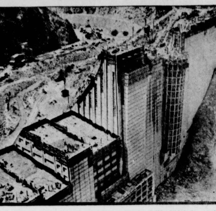
A general view of the huge dam at Azusa, Calif., which is nearing completion and which, when finished, will provide an additional supply of stored water to the city of Pasadena. It will be one of the largest dams in the country, of modern design and earthquake proof. The new dam is 829 feet high from foundation to crest. Its length at the crest is 800 feet, and its thickness at the foundation, 270 feet.
