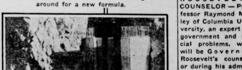
DAM STARTED —With the turbulent Colorado River now flowing through the diversion tunnel (above), actual construction work on the $165,000,000 Hoover Dam was put under way.
