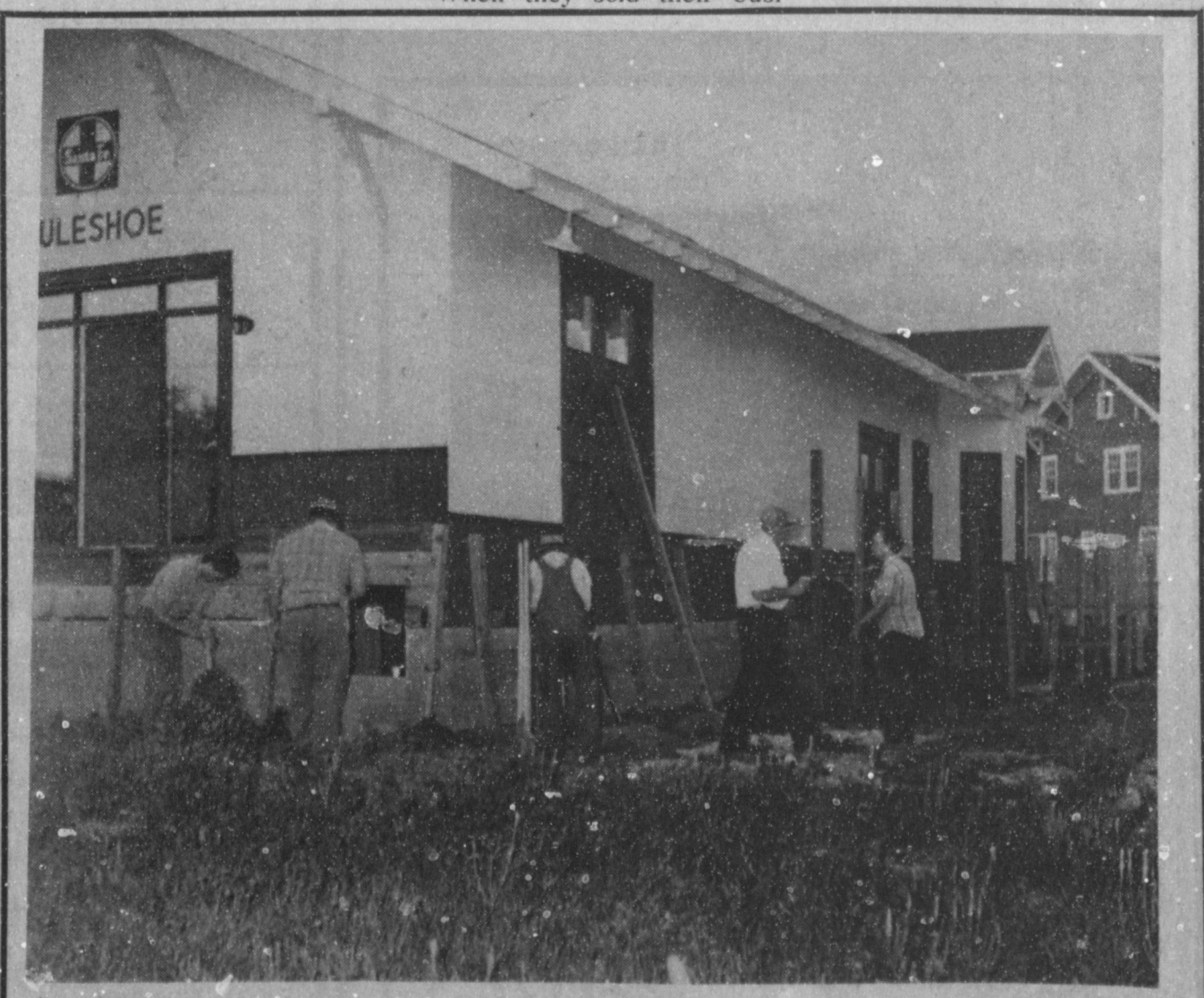
WORKING ON OLD SANTA FE DEPOT --Monday evening, several volunteers were at work, preparing to construct a decking at the Santa Fe Depot building. It is being renovated into a senior citizen center. Shown from left are Phil Kent; Roland McCormick; Carl Ellington; R.A. Bradley and Marie Bradley. Several other men were also working, but not in the picture when it was taken. The final stages of renovation is underway at this time, and the Muleshoe Heritage Foundation is still in need of chairs, table flatware, dishes and cooking pots and pans for the center.
