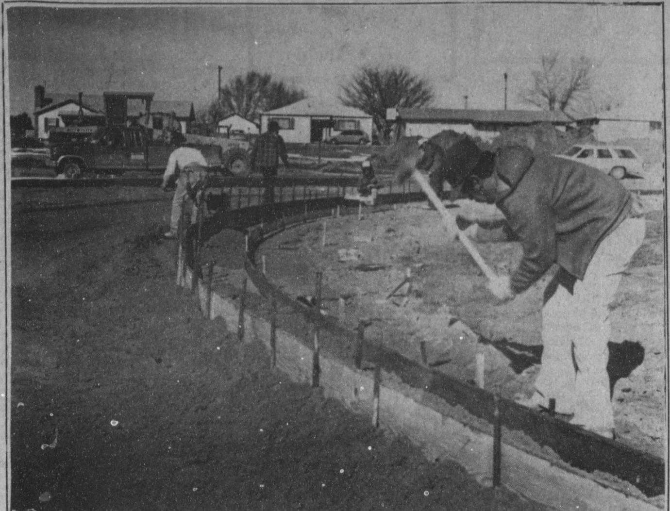
CURB WORK UNDERWAY -Taking advantage of the beautiful days this week, Vela Concrete of Clovis has been busy erecting forms and pouring concrete for the curbing at the new track at Muleshoe High School. J.C. Pearson, of Pearson Construction, and sub-contractors of the new track, said the track construction is running slightly ahead of schedule and the hot mix will be poured by Chris and Tommy Green next month, then the top will be laid by Vibra-Whirl, general contractors for the construction.
