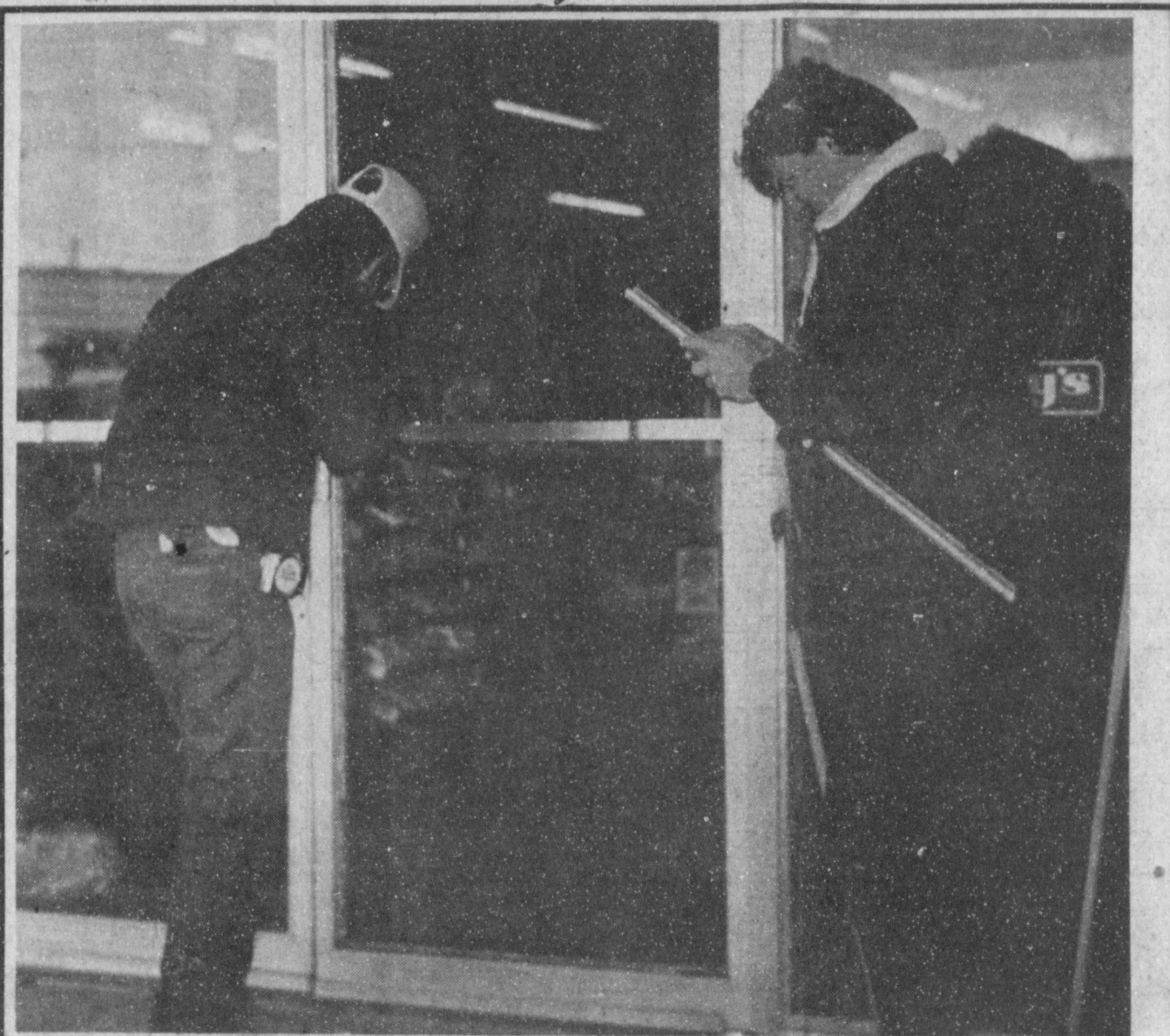
REPAIRING THE DAMAGE - A surprised Linda Foshee, manager of Perry's, arrived at work Monday morning to find the front door of the store broken out and at least $1,000 in merchandise removed from the store. Here workmen from Lubbock Sash and Door are repairing the broken door. Among the missing items from the store are bicycles and radios, according to the report filed. This is the second time for the front door to be broken out in recent weeks as Sgt. Richard Bonham found the door broken out on Christmas morning, although entry was not gained into the store at that time.
