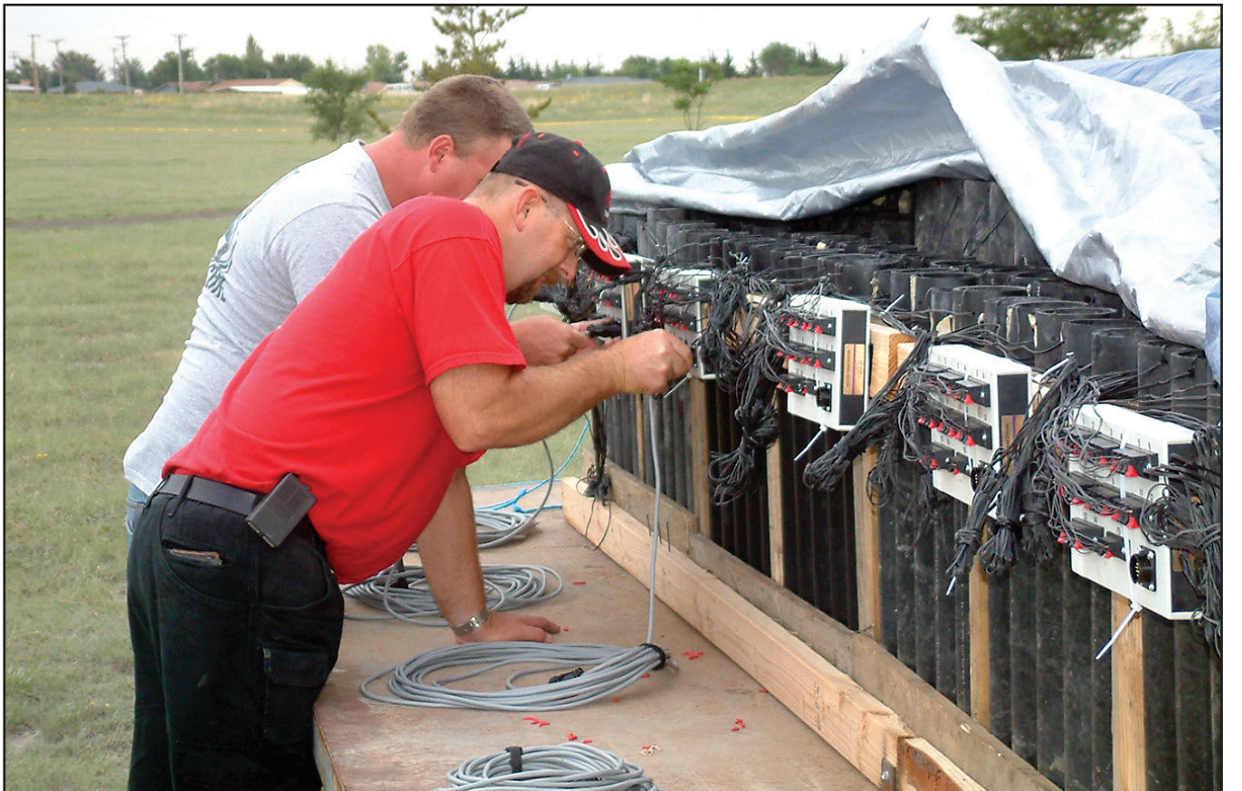
Firefighters Justin Helton and Rick Railsback begin connecting the cables for the fireworks ignition system prior to Saturday's display. The tarp is on hand to protect the equipment and fireworks in the event of rain.
