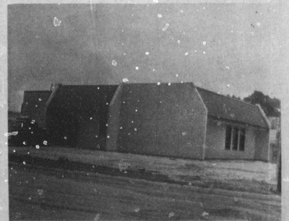
NEW DINING ROOM--Scheduled for completion in the near future is this new addition to the Muleshoe Nursing Home. It will house a dining room, and offices for nursing administrative officials. It is being constructed at the west end of the current nursing home facility, as major renovation of the facility continues.
