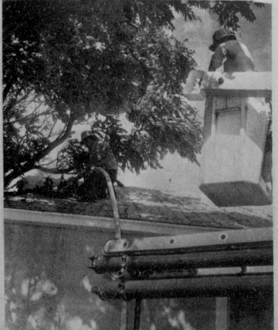
ELECTRICAL FIRE --At mid-afternoon Monday, Muleshoe firemen were summoned to the E.W. Locker home on the West Camp road for a house fire. The firemen found the roof and back of the garage burning, from an apparent electrical short caused by high wind rubbing an electrical line against the garage. No damage was done to the Locker home, just to the garage area.
