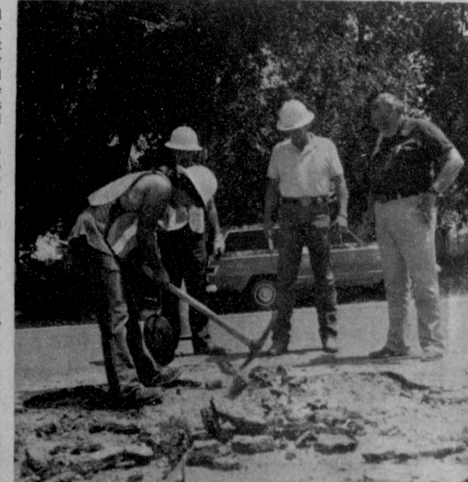
CHECKING FOR DEAD ANTS --Employees of the Texas Department of Highways and Transportation were busy digging up FM2079 in various locations Friday afternoon checking for dead ants in red ant beds. At far right, looking on is Biologist Charles Evans.
