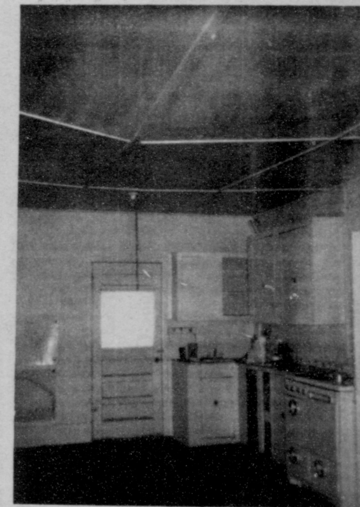
SAGGING Ceiling Needs Cabinet doors on bottom.
