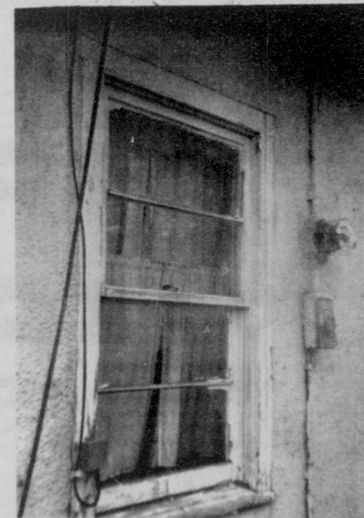
BROKEN Panes & Needs Paint
