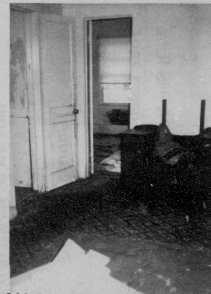
Old carpet partially Removed - peeling Paint. Old furniture
