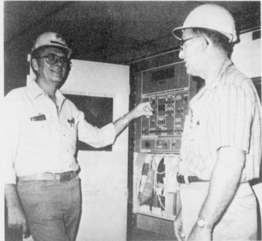
BOILER CONTROL COMPUTER ---Gene Bernhardt, Controls Superintendent, of Muleshoe and J.O. Wimberley, Technician of Littlefield are shown here with the Unit 1 Boiler Control Computer at Tolk Station.
