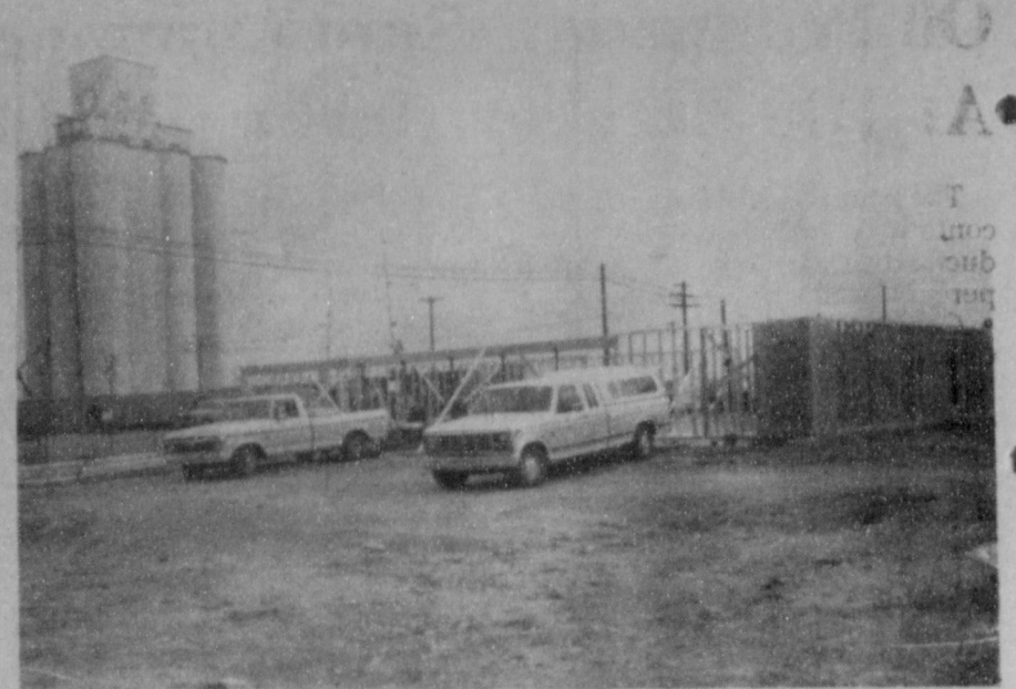
CONSTRUCTION UNDERWAY ---The walls started up this week on the new Town and Country Convenience Store located at the crossroads, of Highway 70 and 84.
