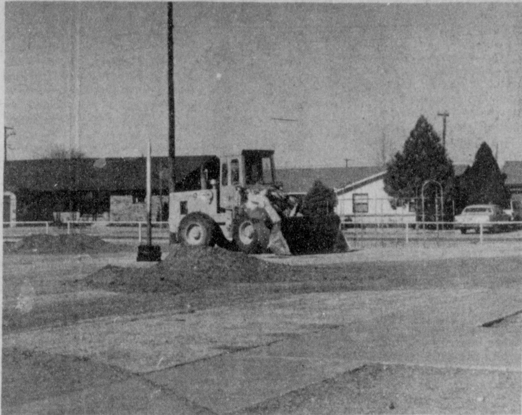
WORK UNDERWAY ON NEW BUILDING... Dirt work began Monday, February 6 on the new activity building at Dillman Elementary. Preliminary work should be finished this week. Estimated time of completion of the building by A&M Builders is two weeks. This building will provide a covered play area for Dillman students.
