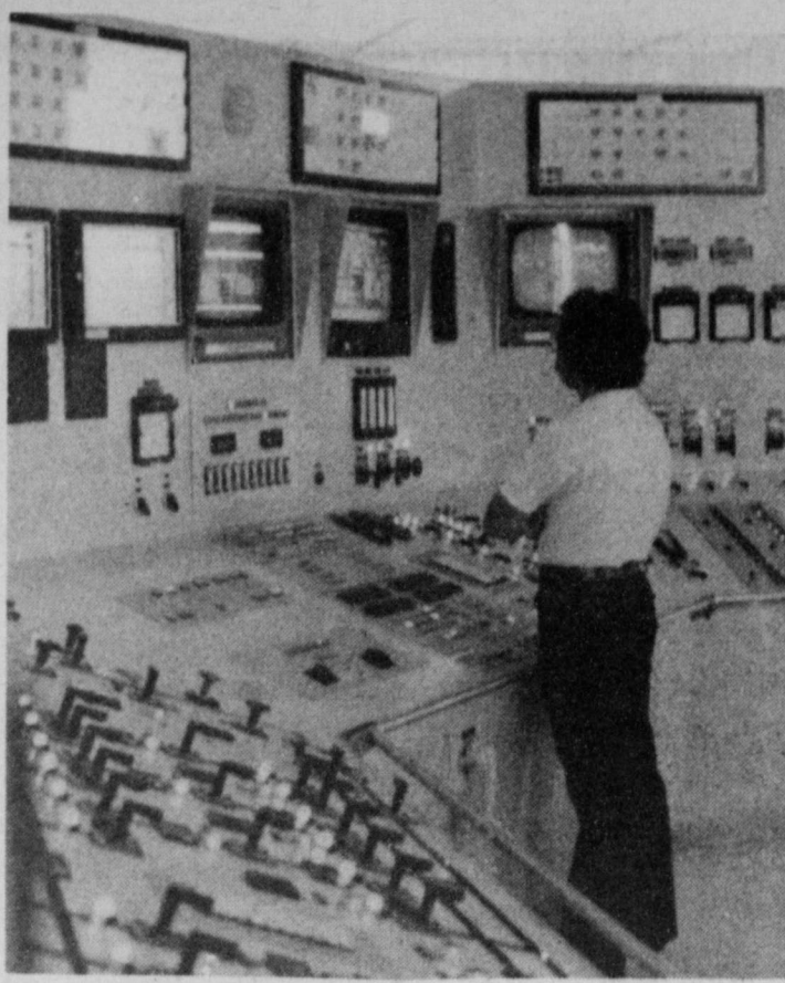
A WATCHFUL EYE--Carlos Saldiver, a control room operator surveys the control 'BTG' board, which is manned 24 hours daily. Every operation in the huge power plant is operated under the eye of the control board and trouble can be spotted as soon as it occurs by a glance at the board.
