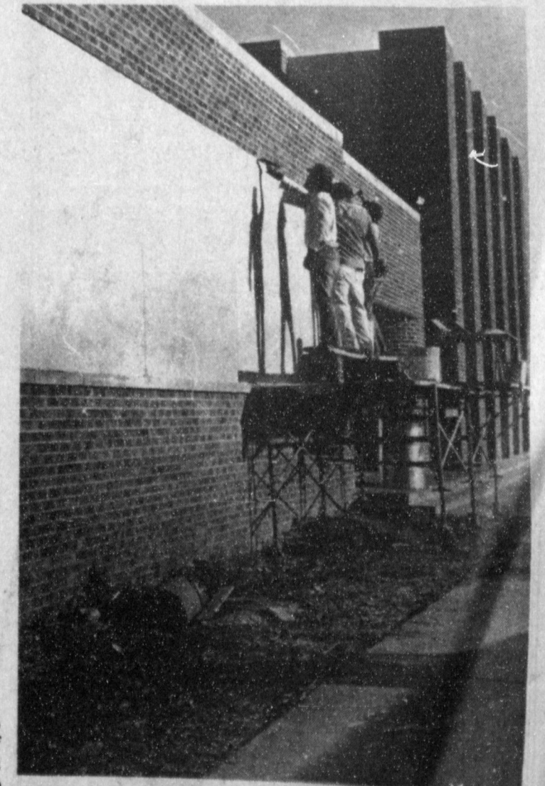
HIGH SCHOOL RENOVATION WORK—Workmen have been busy lately closing up existing windows at the high school and installing heating and insulation as well as lowering inside ceilings. The improvements will help to make the high school look more modern and be more energy efficient, according to studies that have been made.
