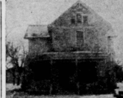
Old house, bottom, became "new" house, top, after it was remodeled by its owner, Kansas wheat farmer Dennis Haines. New roof of asphalt shingles and new windows of ponderosa pine help give the house its modern look.
