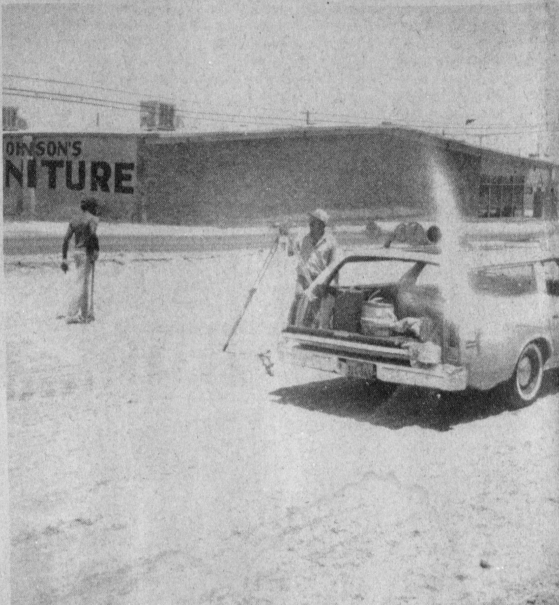
SURVEYING THE HIGHWAY.... After large machinery cut out and removed the south portion of Highway 84 near the west city limits, highway surveyors were checking out levels before a new highway is installed. When the south side is completed, workmen will tear out and rebuild the north two lanes of the highway.
