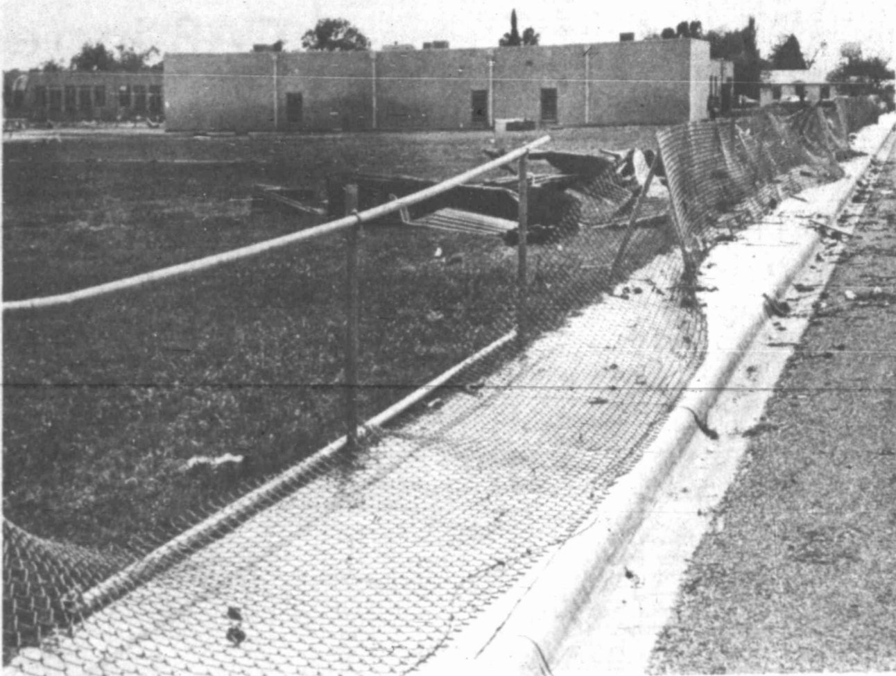
A ripped-off fence is one of several signs of damage at Edwards Elementary School in Monahans, the only school damaged by the tornado which struck the city Tuesday afternoon.
