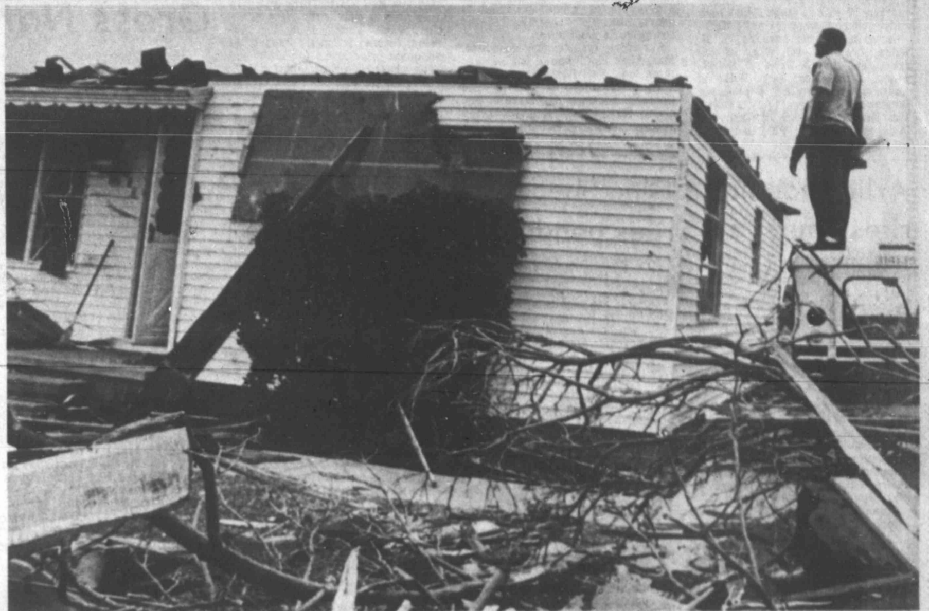
A Monahans postman looks at the damage to his roof from the top of his truck. (Staff Photo by Jim Steinberg)
