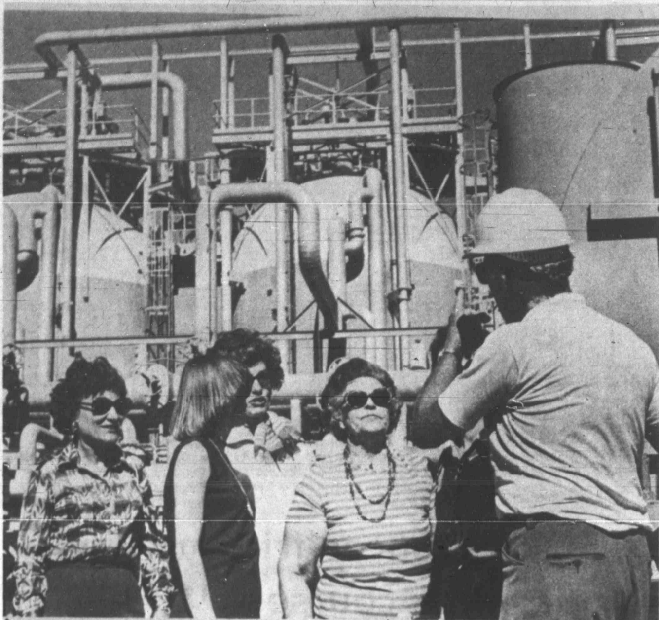
Members of the University Lands' staff in Midland listen as George Richardson, manager of Texas Gulf Sulphur's Comanche Creek mine, explain functions of the tanks and pipe network at the plant that processes raw sulphur. From left are Mrs. Joanna Webb, secretary; Mrs. Phyllis Sellers, production analyst; Mrs. Charlene Hut-
