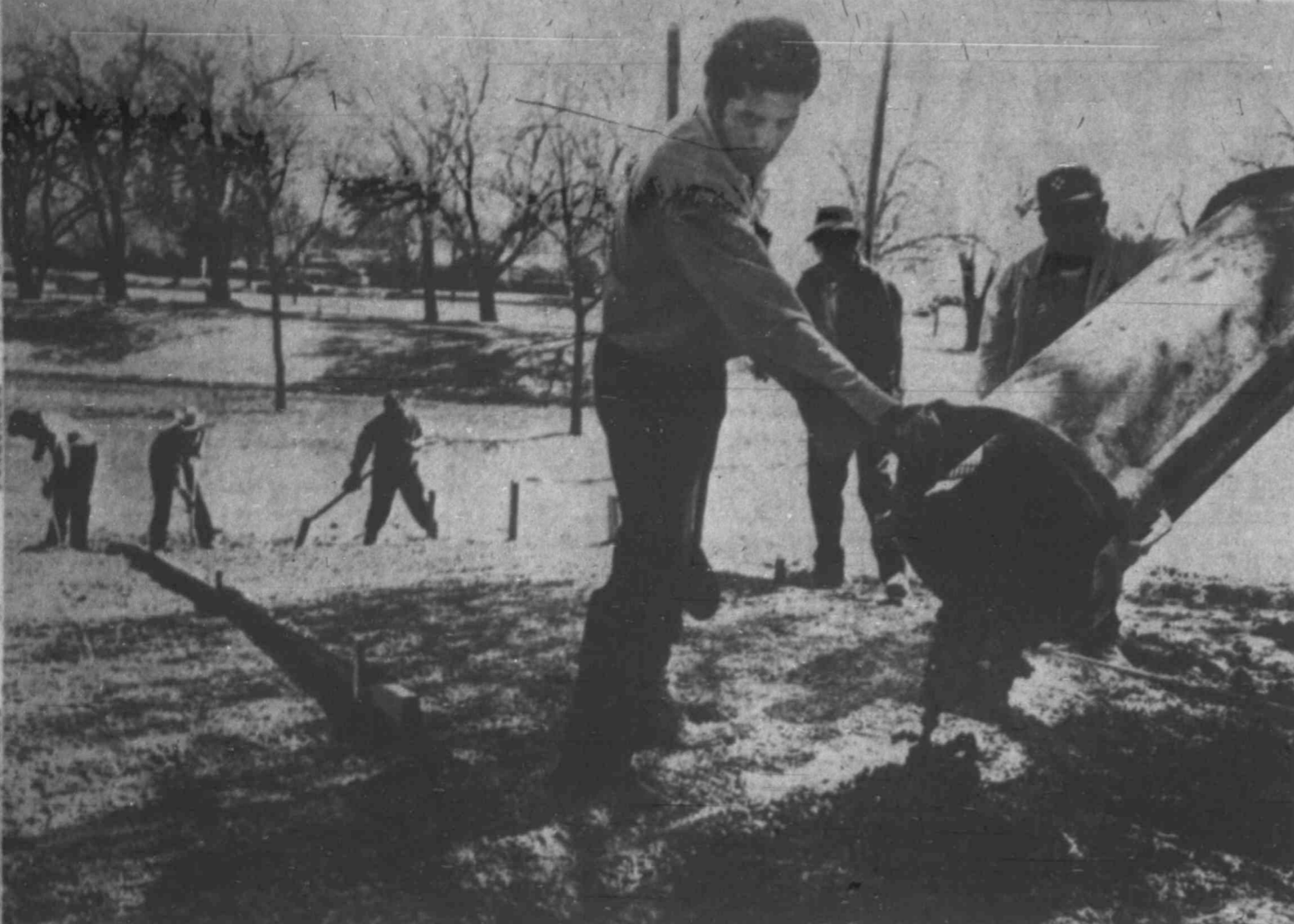
MIDLAND CITY workers pour on the concrete at Wadley-Barron park Tuesday, creating a water-runoff channel into the park. The slab and a retaining wall were added on the park's west side to stop erosion around a large tree. (Staff photo by Bruce Partain).
