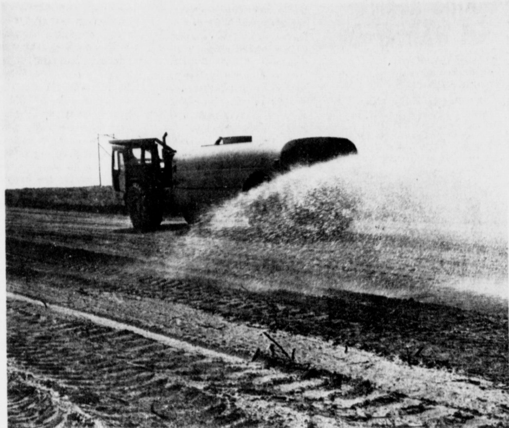
PREPARING A WORKSITE...Stopping the sand from moving around is a large water truck spraying one of the construction sites at Tolk Station, the coal-powered electric generating station east of Muleshoe. Southwestern Public Service Company is constructing the new plant.
