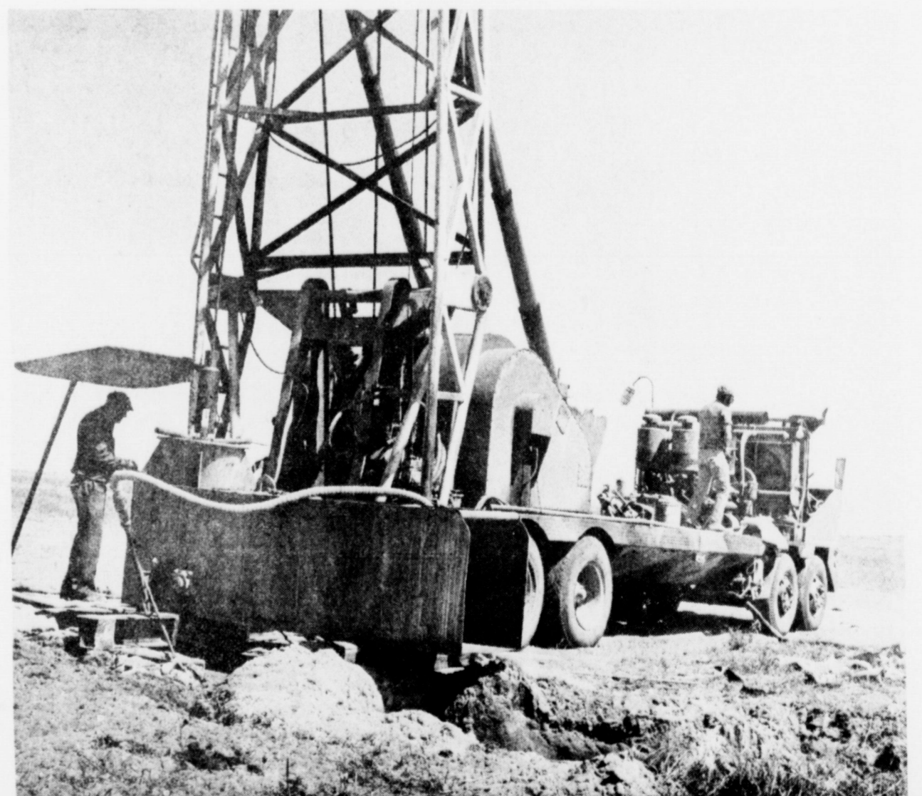
DRILLING AT TOLK PLANT... In mid-year, water well drilling was underway at the location of the new Tolk Station electric generating plant being constructed 10 miles east of Muleshoe by Southwestern Public Service Company. Roads were cut into the area, fences erected and several buildings constructed before the end of 1978. Plant construction is expected to continue for some five years.
