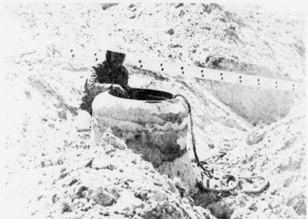
FROM SANDHILLS TO HOMES... Development got underway on the New Parkridge Addition to Muleshoe, just south and west of the city park in southwest Muleshoe. After workmen installed utilities, such as the manholes being constructed here.
