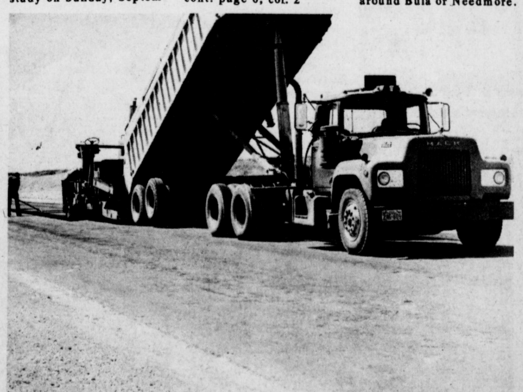
ROAD NEAR COMPLETION...Workmen from Jake Diehl Dirt Moving and Paving were busy this week pouring hot mix on the access road being constructed by Southwestern Public Service to the new electric generating plant site approximately nine miles east of Muleshoe. The road is from the plant site to the SPS property line. An all-weather adjoining road has been completed. Road work was expected to be completed today (Thursday) and workmen will be moving immediately into the area to construct the multi-million dollar plant.
