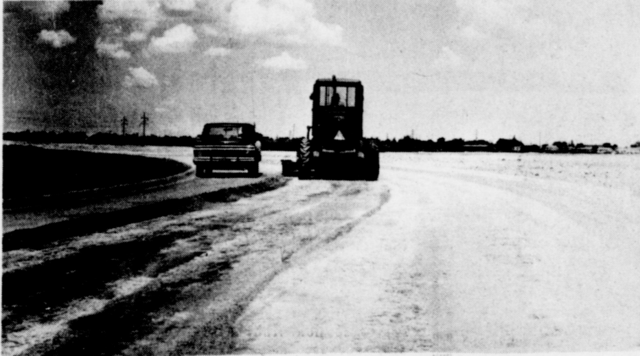
CURBS AND GUTTERS INSTALLED... K. Barnett of Clovis has installed curb and gutter along new streets in the Park Ridge Addition in southwest Muleshoe. In the near future, the Addition will be opened for the construction of new homes. Sewer lines and water mains have already been installed, with electrical and telephone cables being placed underground.
