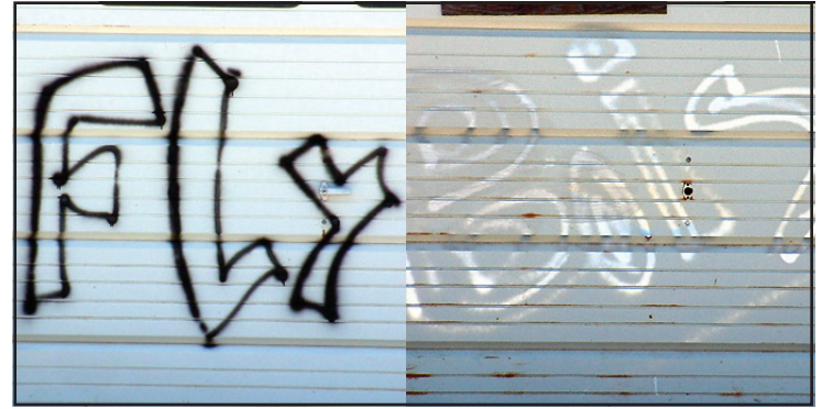
Vandalism on West Ave. B
