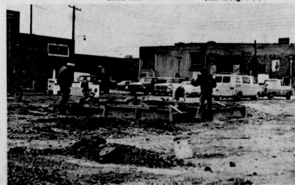
NEW CONSTRUCTION —Poyner's White Stores are in the process of constructing a 40 x 40 building as a warehouse facility and service department for automobiles. Haney Poyner said the metal building will be completed in approximately 90 days. The service department will do tune-ups, front end alignment, wheel balancing and general car repair he said. It is located across the alley east of the present store.
