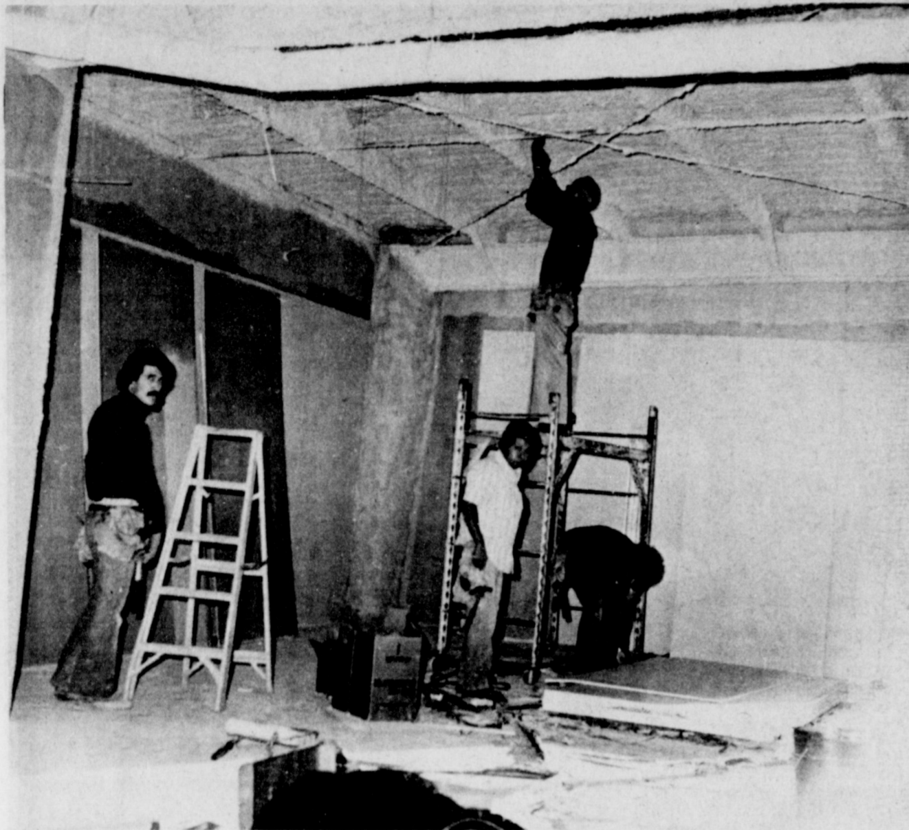
INSULATION GOING ON —These workmen are insulating the Bailey County Civic Center and Coliseum in preparation to putting up the ceiling in the front portion of the new civic center. After getting off to a late start, the work is going along well in construction of the
