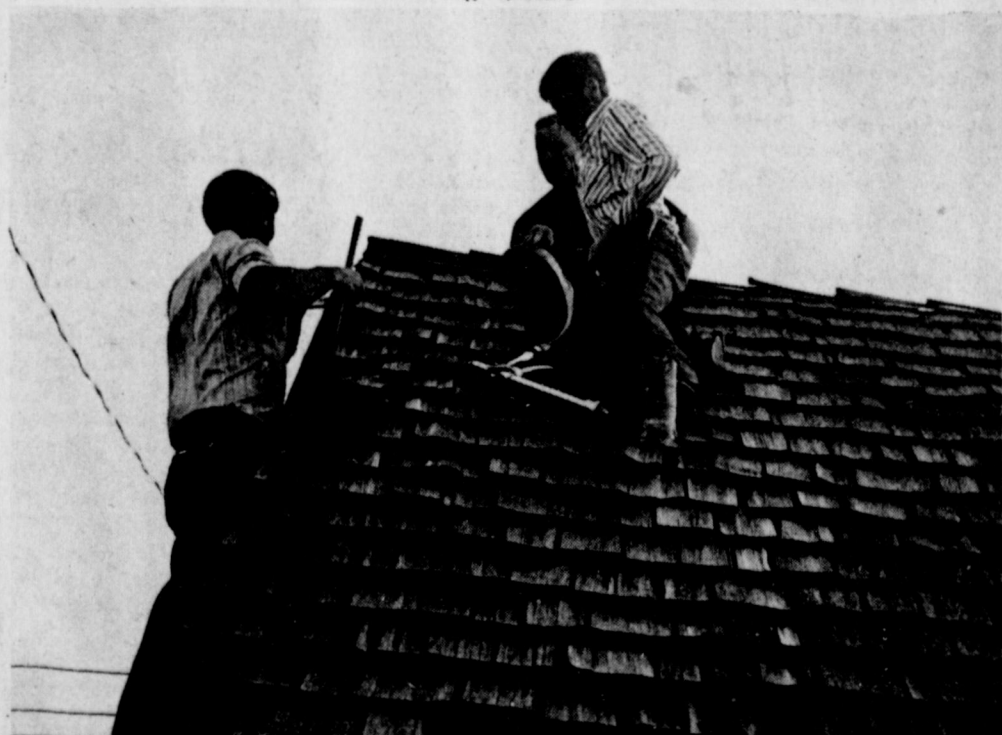
STORM CAUSES FIRE AT CORRAL...A fire was spotted at 8:30 Tuesday morning on top of the Corral Restaurant by a good samaritan a block away who saw smoke coming from the top of the building. The fire was apparently caused by a wire that had broken in the neon tubing around the building and been blown up on top of the roof by the storm the night before. According to Roy Dyer the building suffered some smoke damage and other damage was comparatively light. He stated that they got the people out safely and it had not affected business at all.
