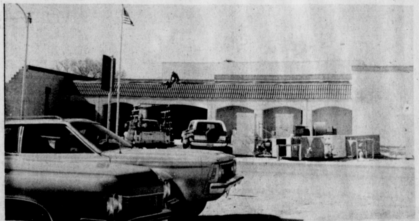
HOSPITAL WORK CONTINUES . . . Workmen have taken advantage of beautiful South Plains weather to rush construction of the new West Plains Medical Center. Here, a workman is installing tile along the front of the new hospital, which is expected to be
