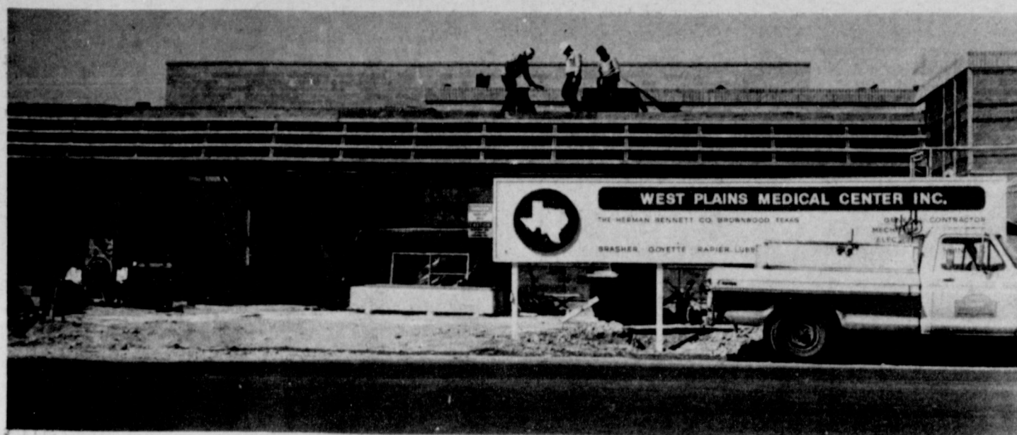
HOSPITAL WORK PROGRESSES . . . Walt Price, general superintendent of the construction of the new hospital facility in Muleshoe said the work is running ahead of schedule on the new portion of the hospital and occupancy is expected early in
