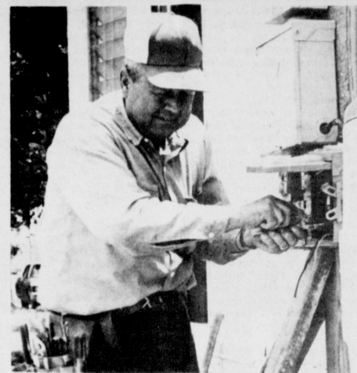
ELECTRICIAN AT WORK . . . Curtis Chapman, electrician from Lubbock, will be in charge of electrical work done on the new hospital in Muleshoe just getting underway this week. Chapman said all electrical systems will be thoroughly checked by him before final approval for hospital use.
