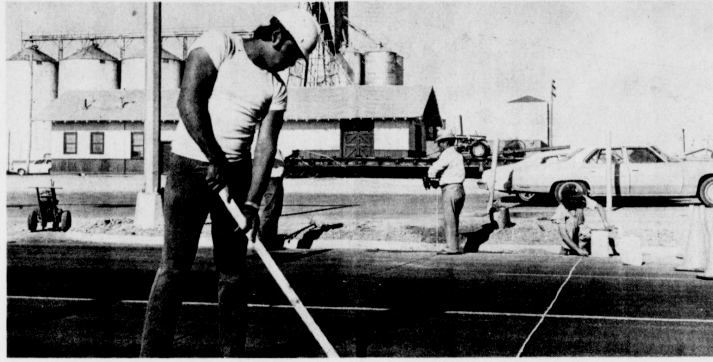
TRAFFIC SENSORS INSTALLED . . . Wiley Melton, Jerry Chancellor and Richard Seideman of the Department of Highways and Public Transportation from Lubbock and Joe Cuellas of Muleshoe are shown installing traffic sensors or loops which will record the amount of traffic flow into the intersection of Main and American Blvd.
